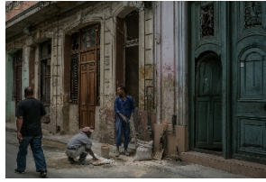
Workers preparing sand during the renovation of a compound in the old section of Havana. Credit Mauricio Lima for The New York Times
