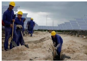
File photo: workers install a high-voltage power line that will carry the current generated by solar panels at Cuba's first solar farm in Cantarana. New regulatory changes would allow U.S. engineering and design firms to work on such infrastructure projects in Cuba. Franklin Reyes AP
